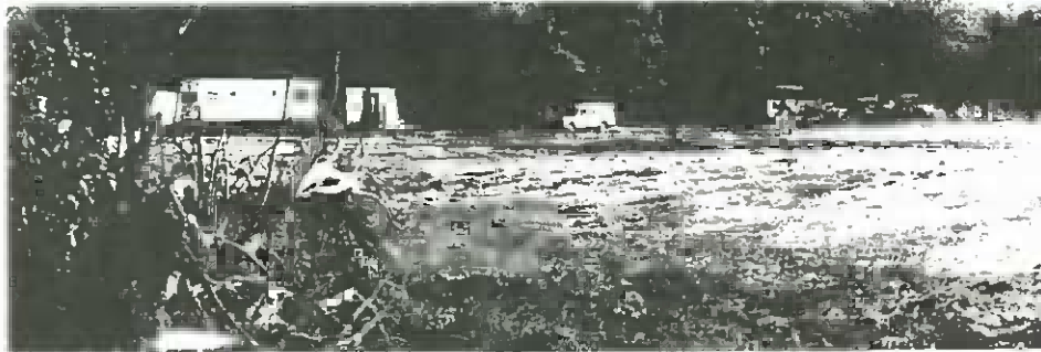
FIRST STEP — An empty field is all one sees of the new Hostess House which will be built next to the bank on Holcomb Blvd. Members of Daniec Construction Company, Jacksonville, Fla.,
