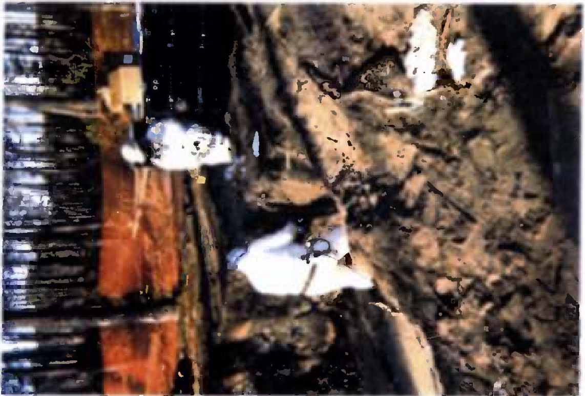
Project No. 15226 Contract No. N47408-92-D-3042 Delivery Order: 32 Location : Description: confirmation sampling of trenches
