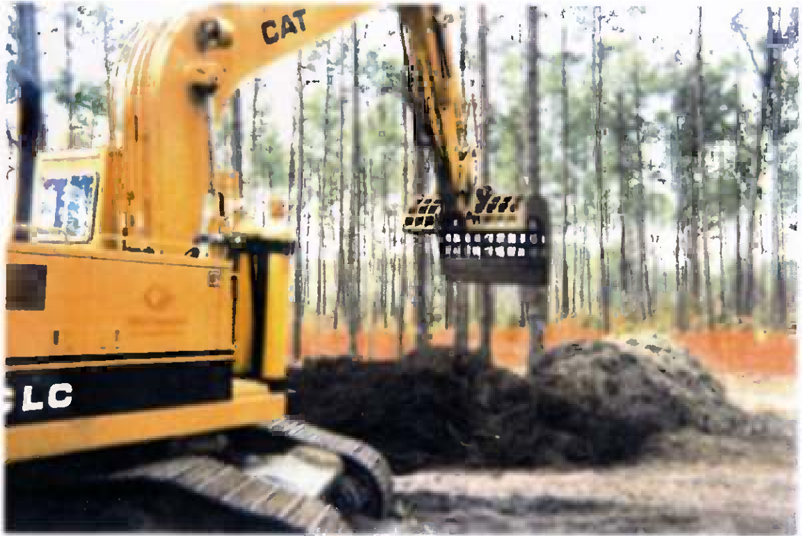
Project No. 15226 Contract No. N47408-92-D-3042 Delivery Order: 32 Location : south trenches Description: removal of debris & batteries from trenches
