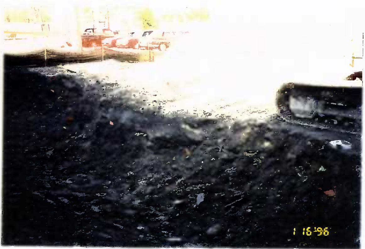
Project No. 17418 Date: 1/16/96 Contract No. N62470-93-D-3032 Delivery Order: 78 Location: Building 25 Description: Location of sample points for composite sample
