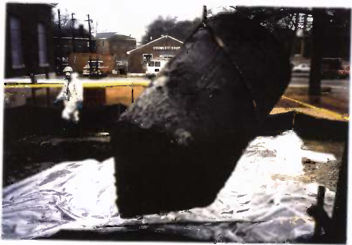
Project No. 17418 Date: 1/12/96 Contract No. N62470-93-D-3032 Delivery Order: 78 Location: Building 25 Description: Removal of UST
