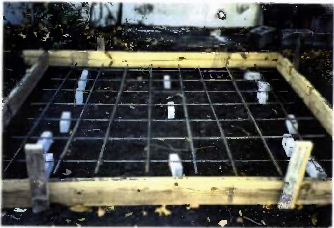
Project No. 17418 Date: 12/14/95 Contract No. N62470-93-D-3032 Delivery Order: 78 Location: Building 25 Description: Form and rebar for air compressor pad
