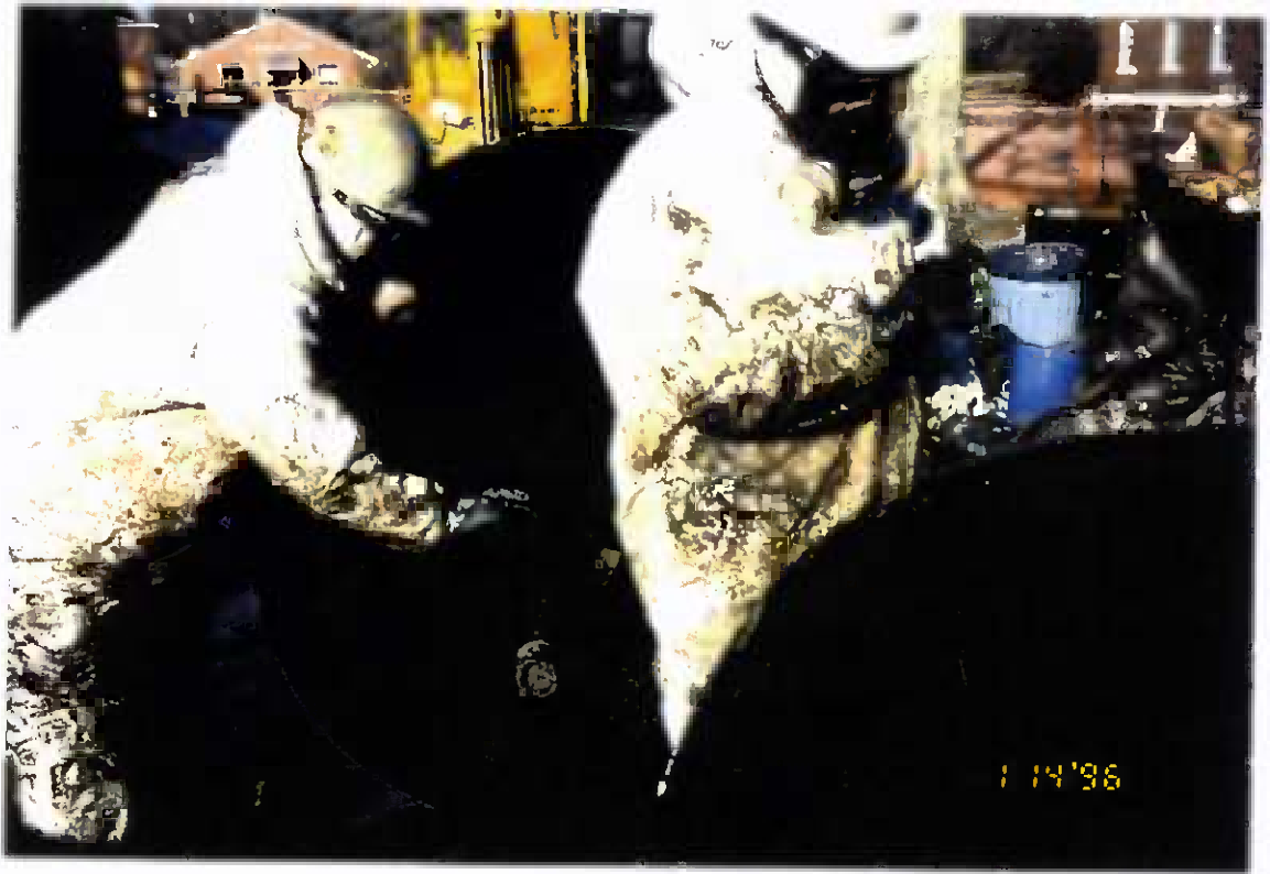
Project No. 17418 Date: 1/14/96 Contract No. N62470-93-D-3032 Delivery Order: 78 Location: Building 25 Description: Demolition of USTs
