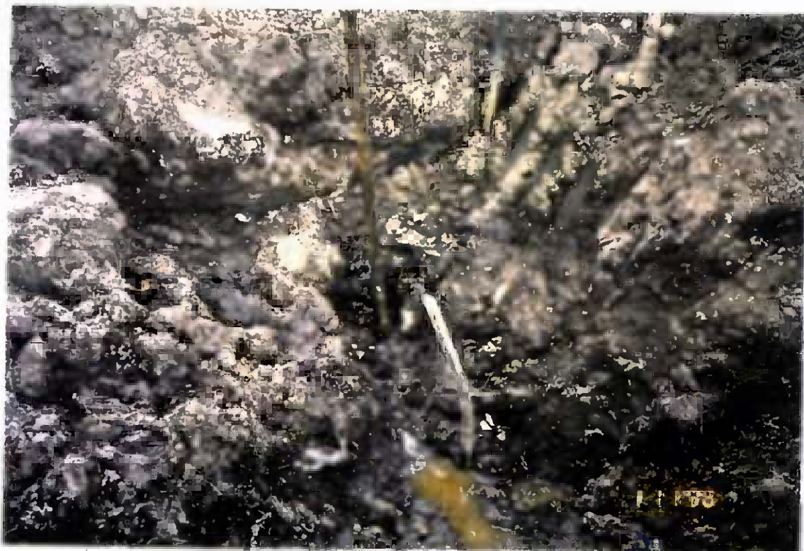
Project No. 17418 Date: 1/11/96 Contract No. N62470-93-D-3032 Delivery Order: 78 Location: Building 25 Description: Tank thief used to remove tank contents
