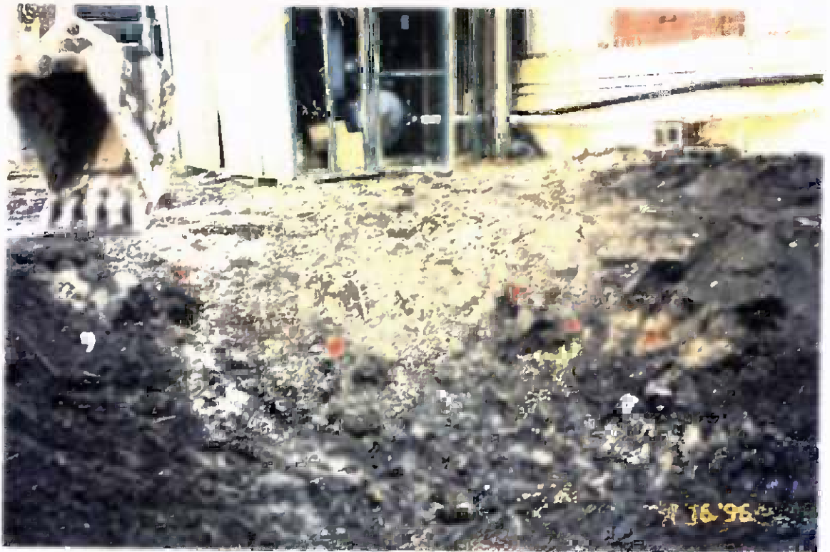
Project No. 17418 Date: 1/16/96 Contract No. N62470-93-D-3032 Delivery Order: 78 Location: Building 25 Description: Location of sample points for composite sample
