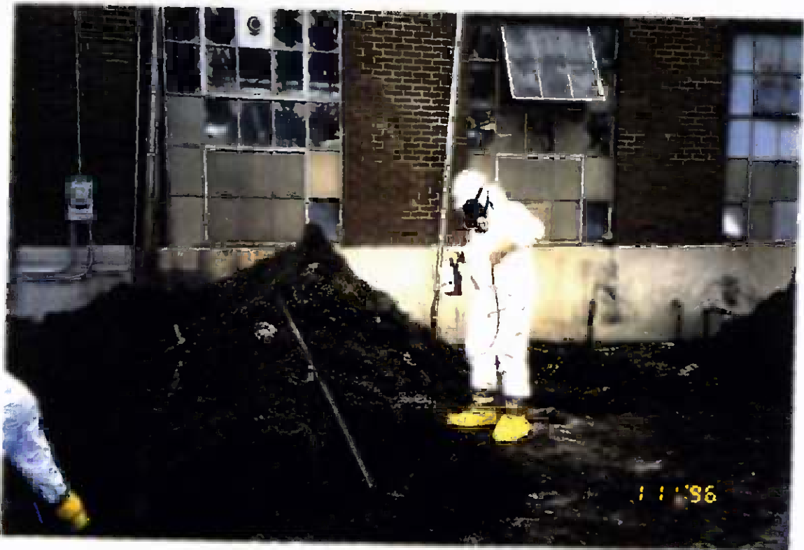
Project No. 17418 Date: 1/11/96 Contract No. N62470-93-D-3032 Delivery Order: 78 Location: Building 25 Description: Air monitoring from the tanks
