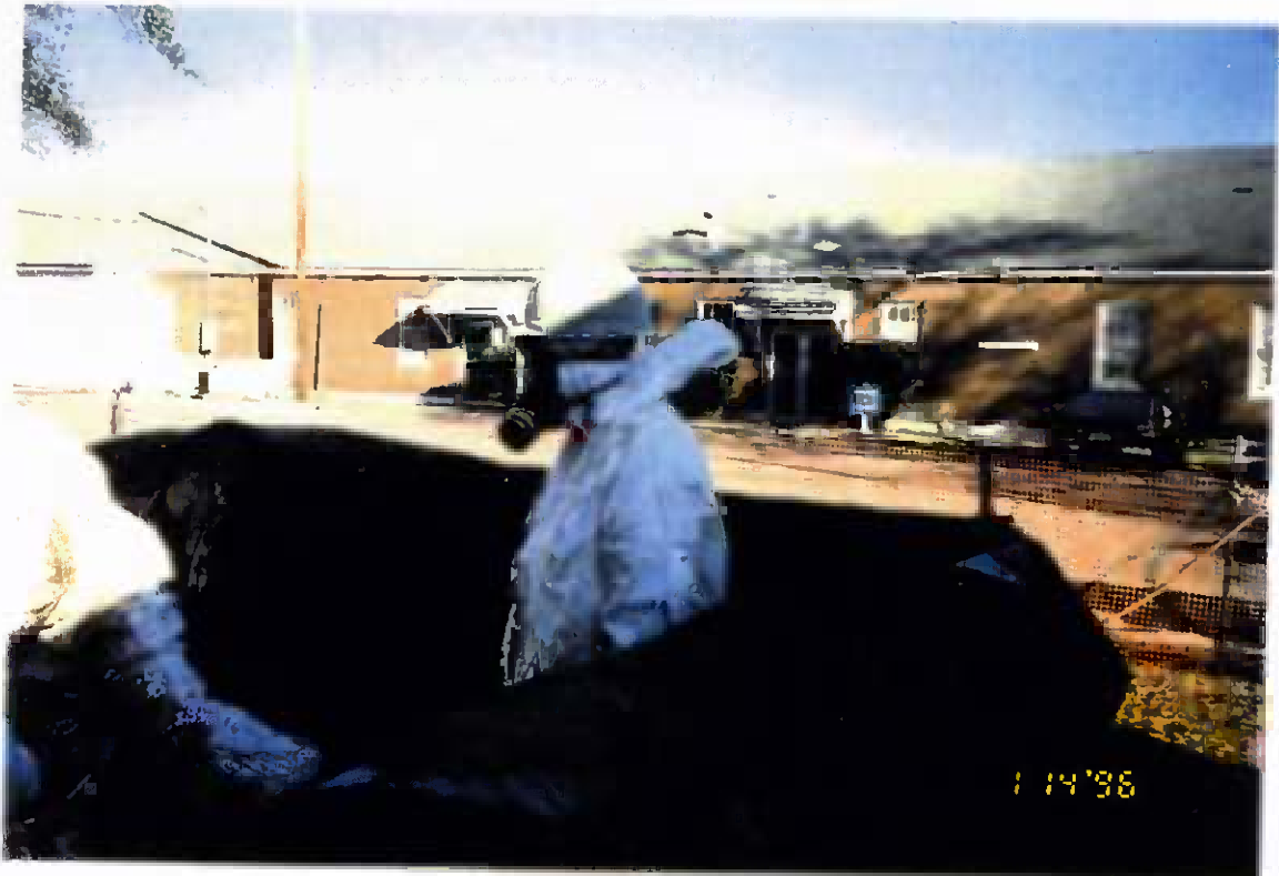
Project No. 17418 Date: 1/14/96 Contract No. N62470-93-D-3032 Delivery Order: 78 Location: Building 25 Description: Demolition of USTs
