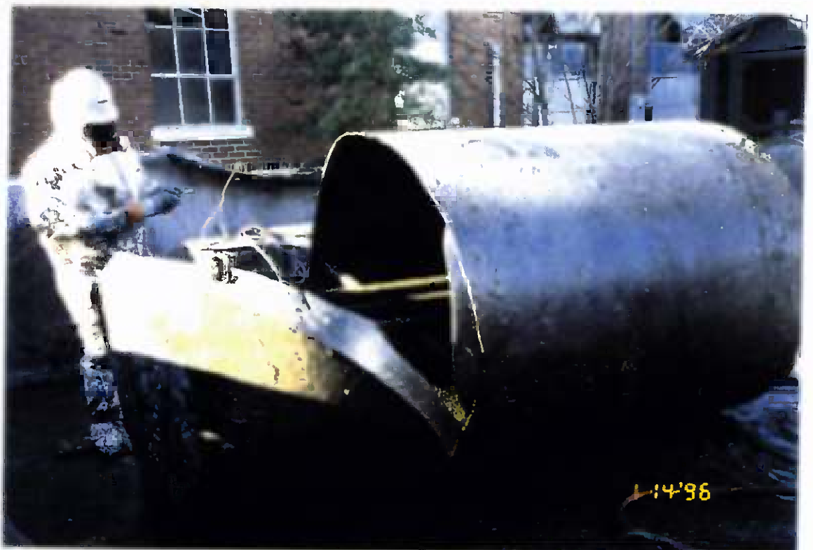
Project No. 17418 Date: 1/14/96 Contract No. N62470-93-D-3032 Delivery Order: 78 Location: Building 25 Description: Demolition of USTs
