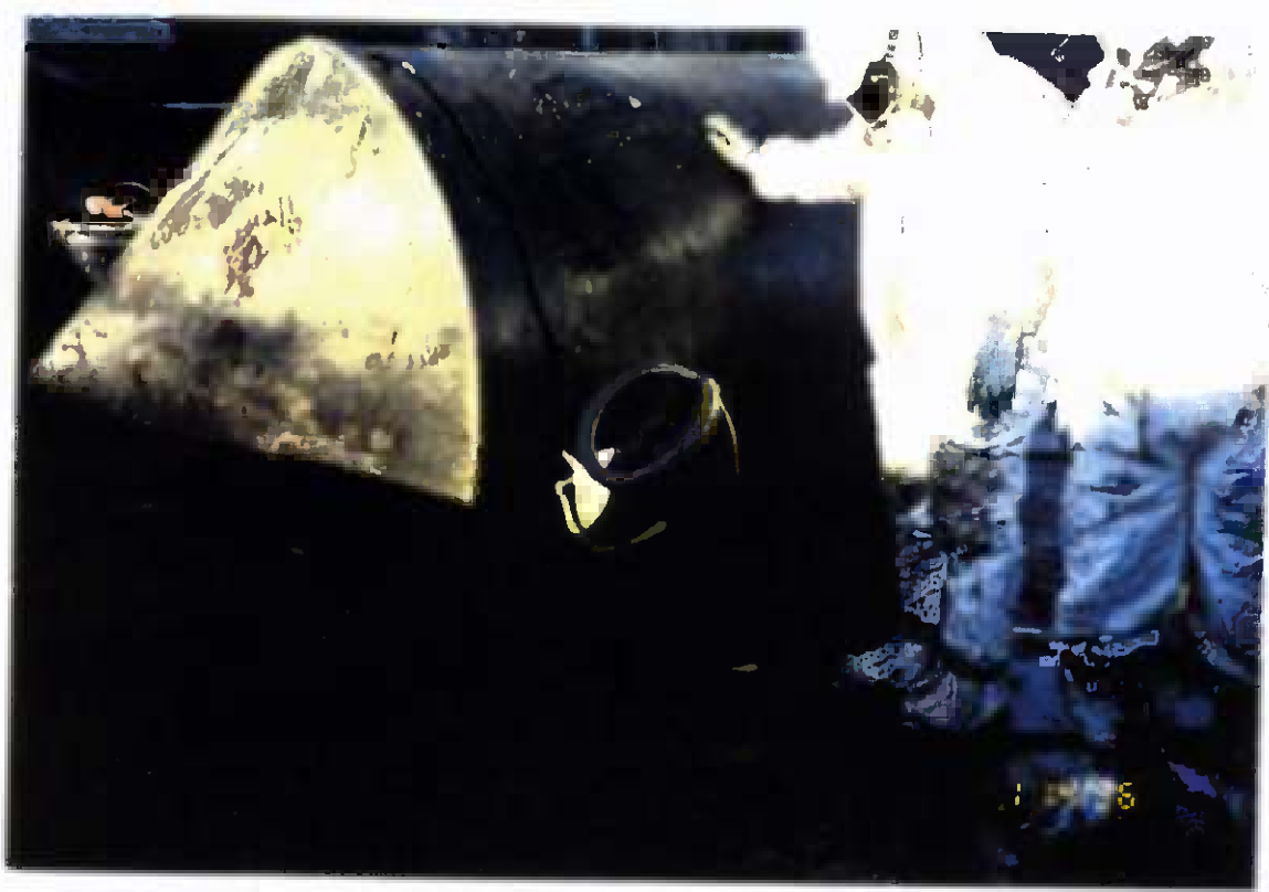
Project No. 17418 Date: 1/14/96 Contract No. N62470-93-D-3032 Delivery Order: 78 Location: Building 25 Description: Cutting of UST with pneumatic nibbler
