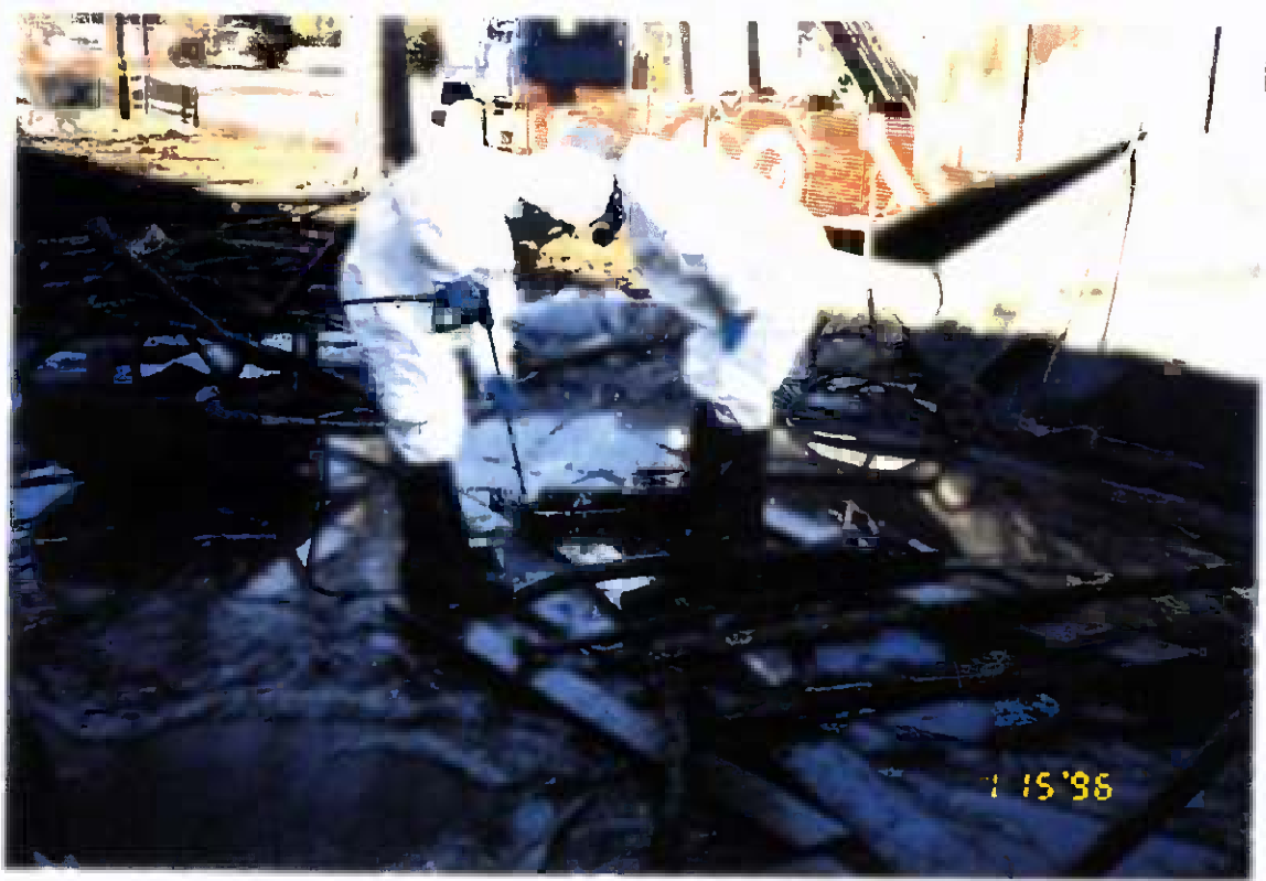
Project No. 17418 Date: 1/15/96 Contract No. N62470-93-D-3032 Delivery Order: 78 Location: Building 25 Description: Decon of piping
