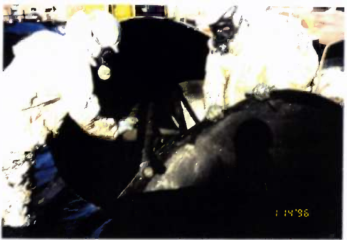
Project No. 17418 Date: 1/14/96 Contract No. N62470-93-D-3032 Delivery Order: 78 Location: Building 25 Description: Demolition of USTs
