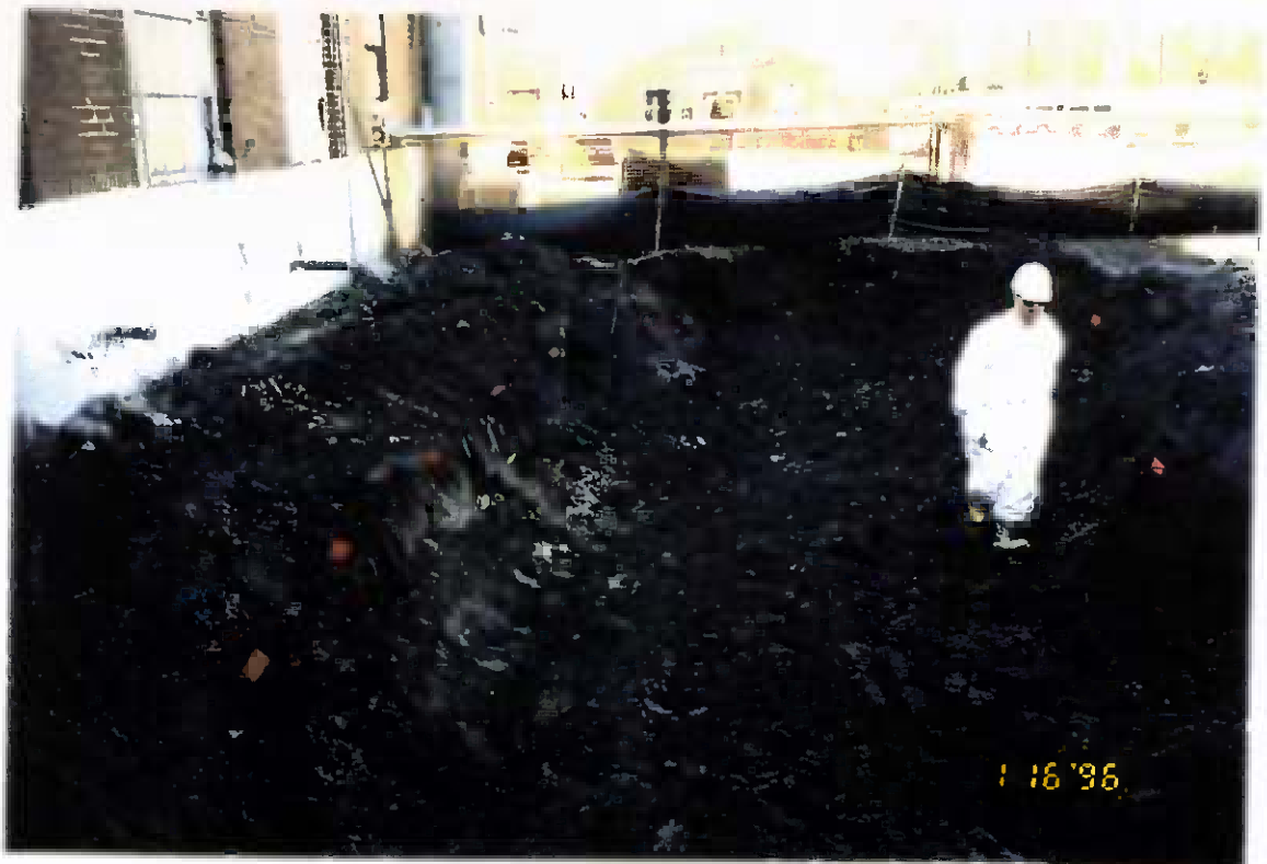
Project No. 17418 Date: 1/16/96 Contract No. N62470-93-D-3032 Delivery Order: 78 Location: Building 25 Description: Location of sample points for composite sample
