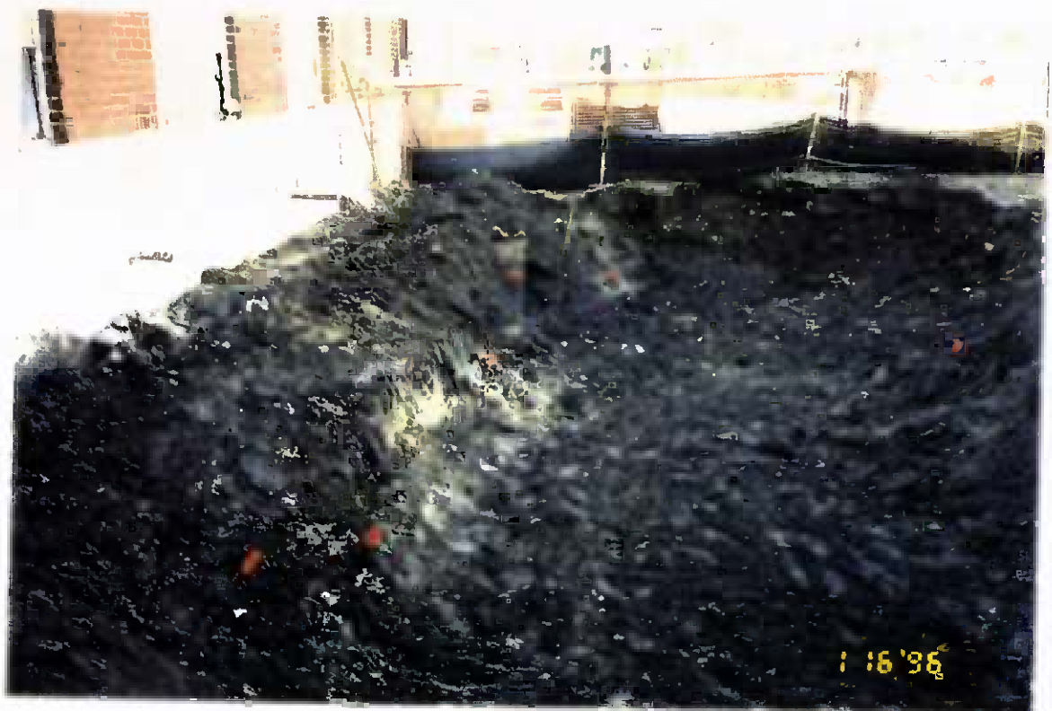
Project No. 17418 Date: 1/16/96 Contract No. N62470-93-D-3032 Delivery Order: 78 Location: Building 25 Description: Location of sample points for composite sample
