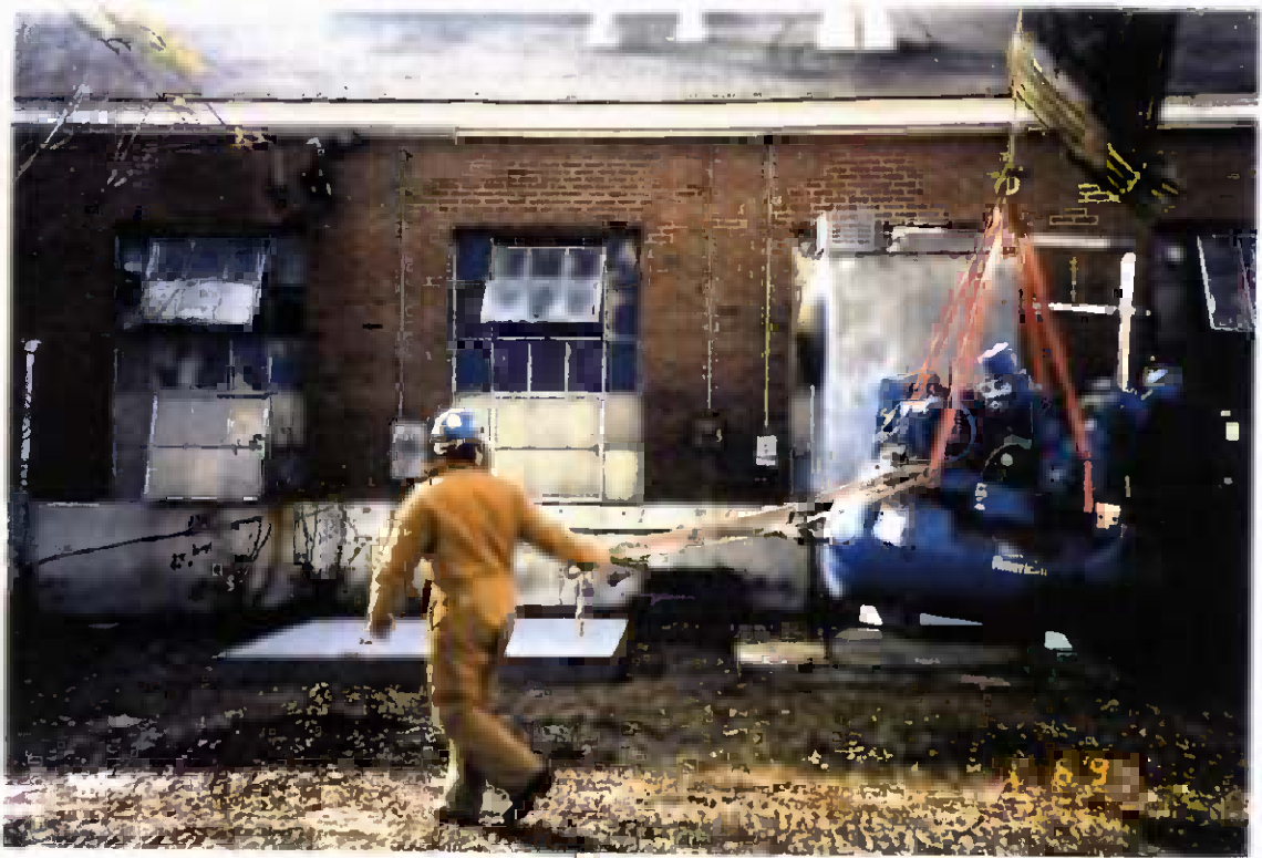
Project No. 17418 Date: 1/6/96 Contract No. N62470-93-D-3032 Delivery Order: 78 Location: Building 25 Description: Relocation of air compressor
