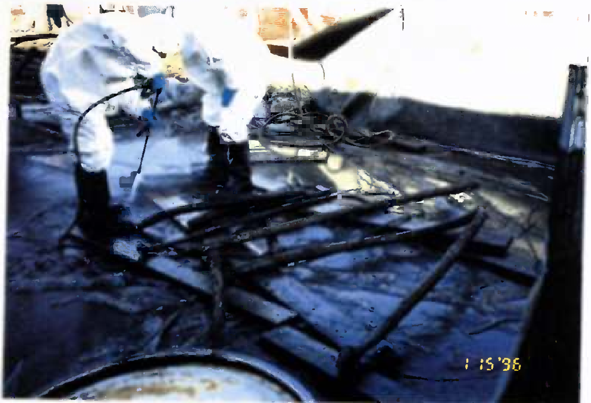
Project No. 17418 Date: 1/15/96 Contract No. N62470-93-D-3032 Delivery Order: 78 Location: Building 25 Description: Demolition of USTs
