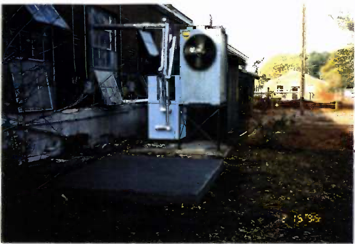
Project No. 17418 Date: 12/15/95 Contract No. N62470-93-D-3032 Delivery Order: 78 Location: Building 25 Description: Pad for air compressor
