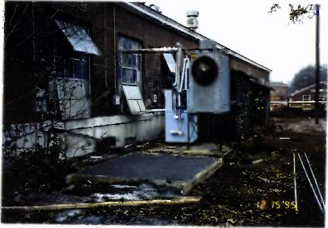
Project No. 17418 Date: 12/15/95 Contract No. N62470-93-D-3032 Delivery Order: 78 Location: Building 25 Description: Pad for air compressor
