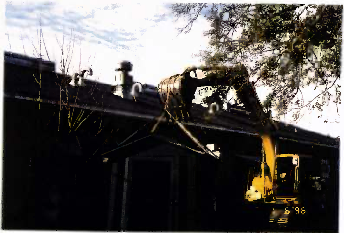
Project No. 17418 Date: 1/6/96 Contract No. N62470-93-D-3032 Delivery Order: 78 Location: Building 25 Description: Relocation of air compressor shed
