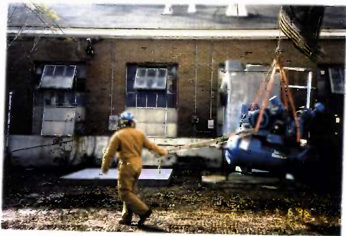
Project No. 17418 Date: 1/6/96 Contract No. N62470-93-D-3032 Delivery Order: 78 Location: Building 25 Description: Relocation of air compressor
