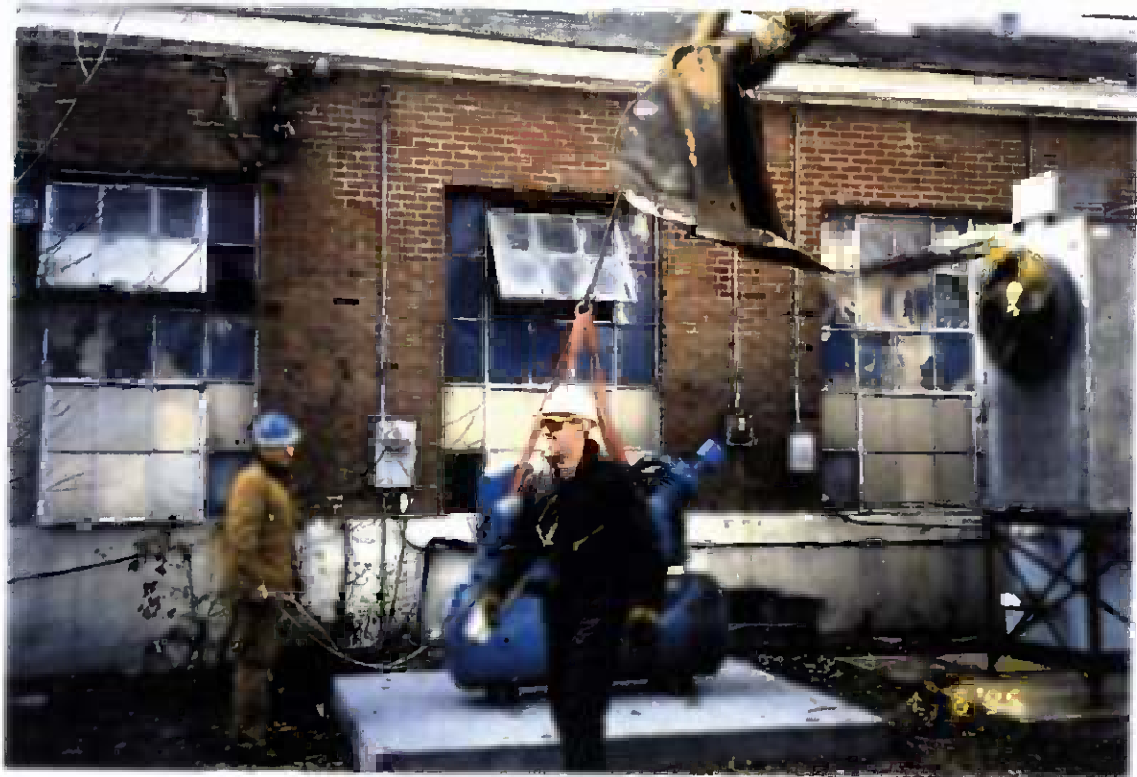
Project No. 17418 Date: 1/6/96 Contract No. N62470-93-D-3032 Delivery Order: 78 Location: Building 25 Description: Relocation of air compressor
