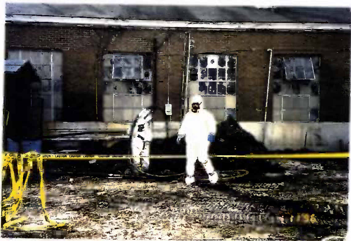
Project No. 17418 Date: 1/11/96 Contract No. N62470-93-D-3032 Delivery Order: 78 Location: Building 25 Description: Removal of tank contents into a tanker truck
