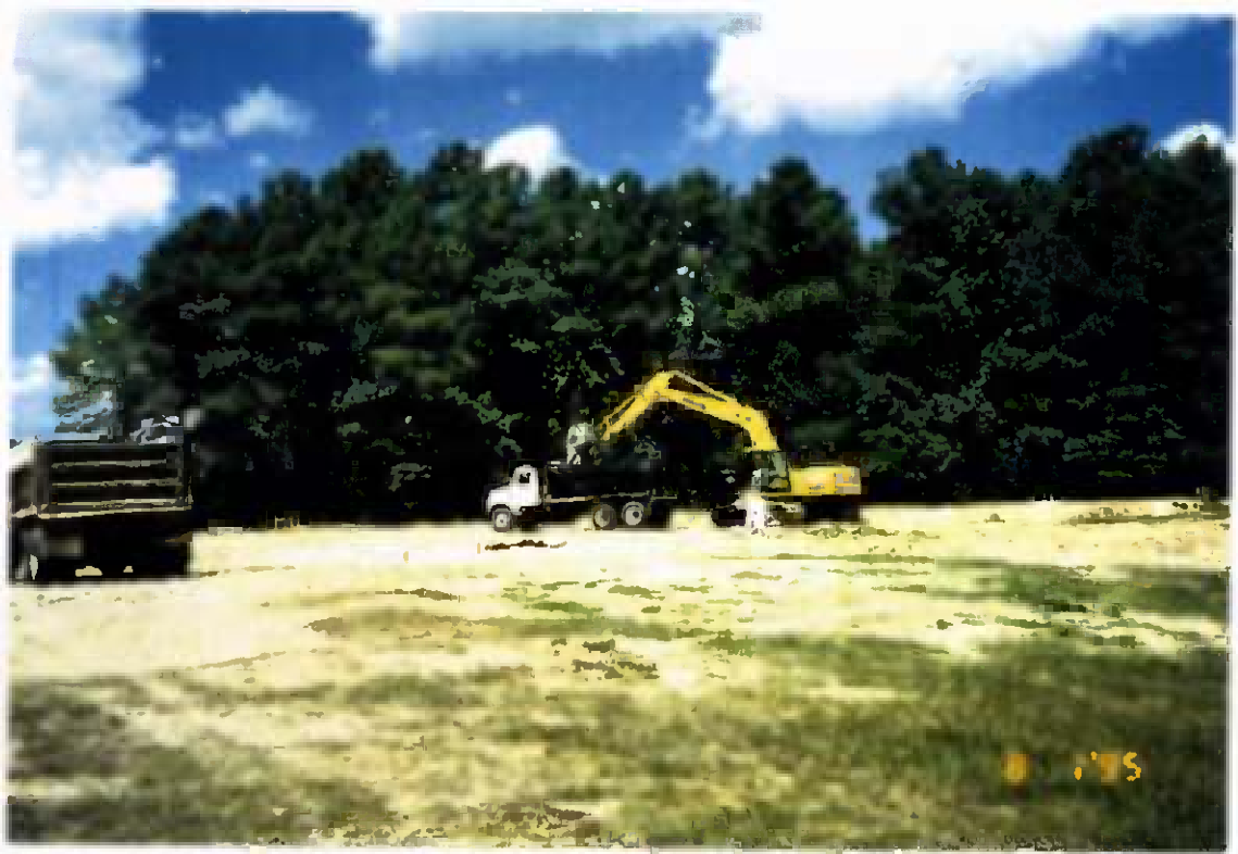
Project No. 16487 Date: 8/1/95 Contract No. N62470-93-D-3032 Delivery Order: 44 Location: Area C Description: Excavating possible TPH contaminated soil
