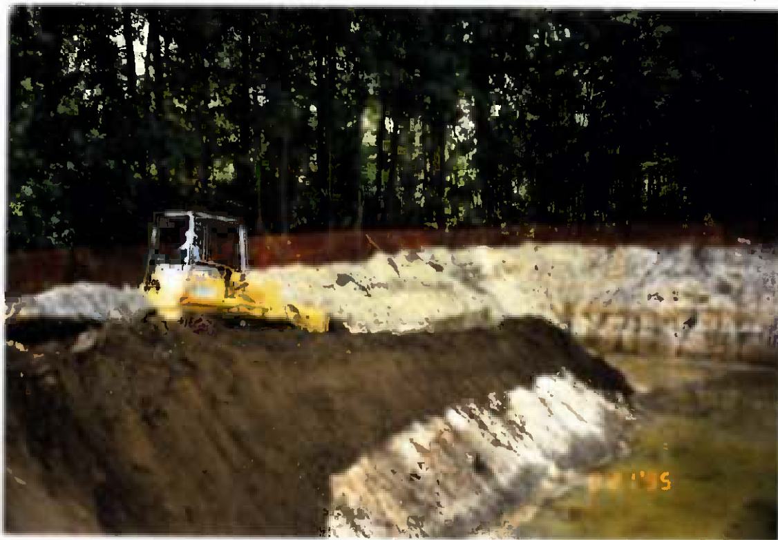
Project No. 16487 Date: 8/21/95 Contract No. N62470-93-D-3032 Delivery Order: 44 Location: Area C Description: Backfilling operations
