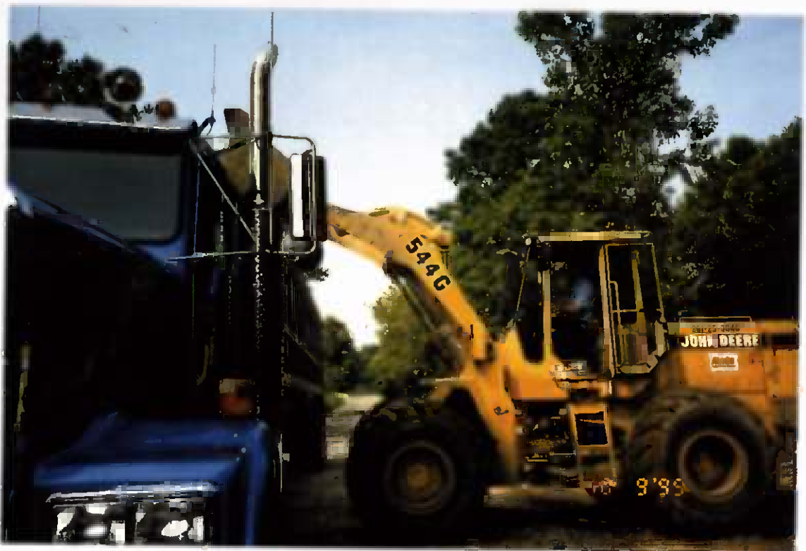
Project No. 16487 Date: 10/9/95 Contract No. N62470-93-D-3032 Delivery Order: 44 Location: Contaminated soil staging area Description: Truck loadout
