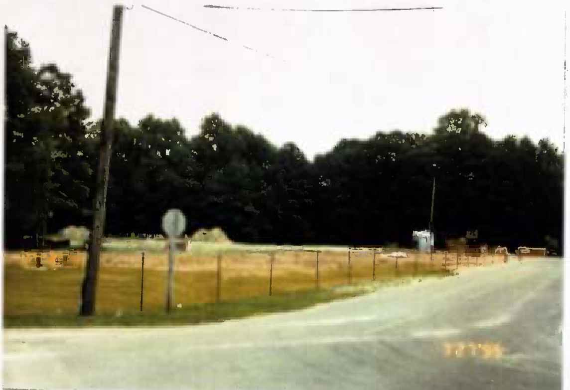
Project No. 16487 Date: 7/27/95 Contract No. N62470-93-D-3032 Delivery Order: 44 Location: Area C Description: Site Prep
