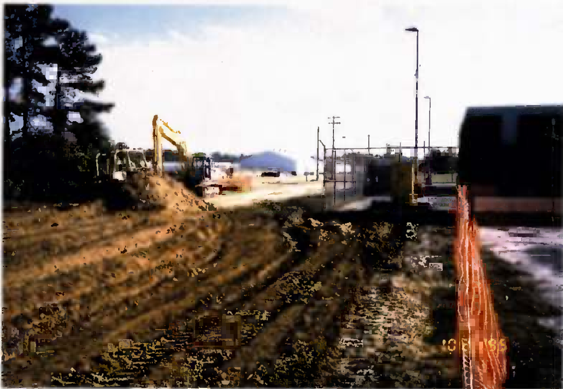
Project No. 16487 Date: 10/24/95 Contract No. N62470-93-D-3032 Delivery Order: 44 Location: Area A Description: Backfill of Area A
