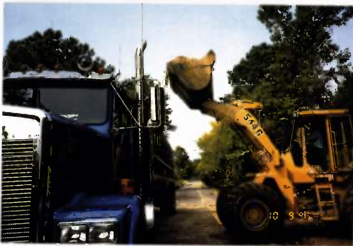
Project No. 16487 Date: 10/9/95 Contract No. N62470-93-D-3032 Delivery Order: 44 Location: Contaminated soil staging area Description: Truck loadout
