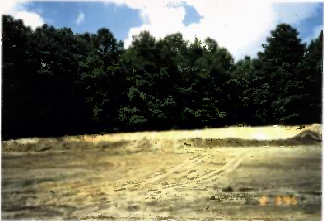
Project No. 16487 Date: 8/3/95 Contract No. N62470-93-D-3032 Delivery Order: 44 Location: Area C Description: Area C excavation
