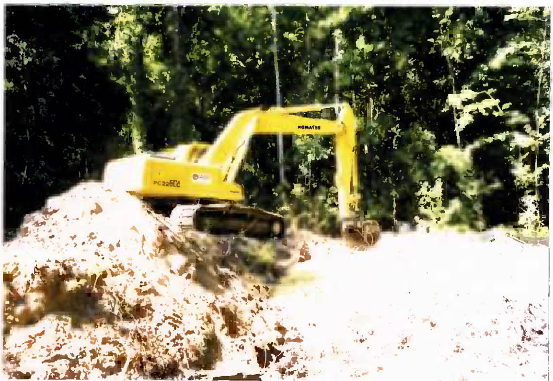
Project No. 16487 Date: 8/9/95 Contract No. N62470-93-D-3032 Delivery Order: 44 Location: Area B Description: Excavation
