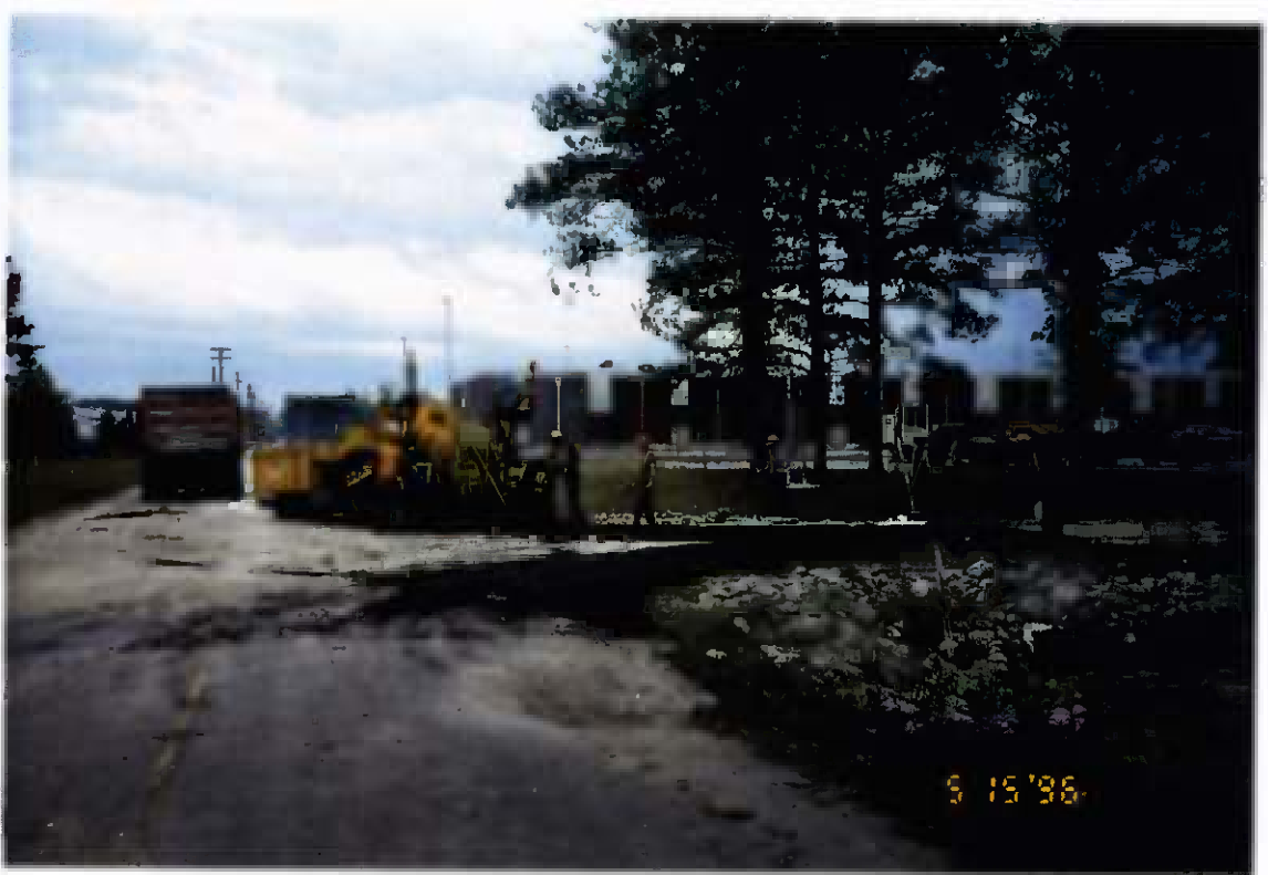
Project No. 16487 Date: 5/15/96 Contract No. N62470-93-D-3032 Delivery Order: 44 Location: Third Street - Camp Geiger Description: Placing asphalt paving
