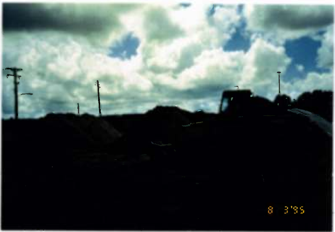
Project No. 16487 Date: 8/3/95 Contract No. N62470-93-D-3032 Delivery Order: 44 Location: Area C Description: Clean soil staging area
