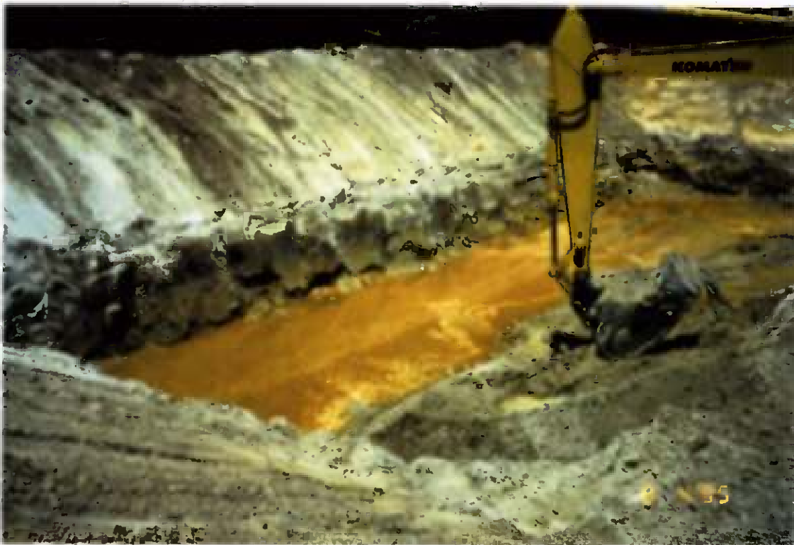
Project No. 16487 Date: 8/4/95 Contract No. N62470-93-D-3032 Delivery Order: 44 Location: Area C Description: Groundwater in bottom of excavation
