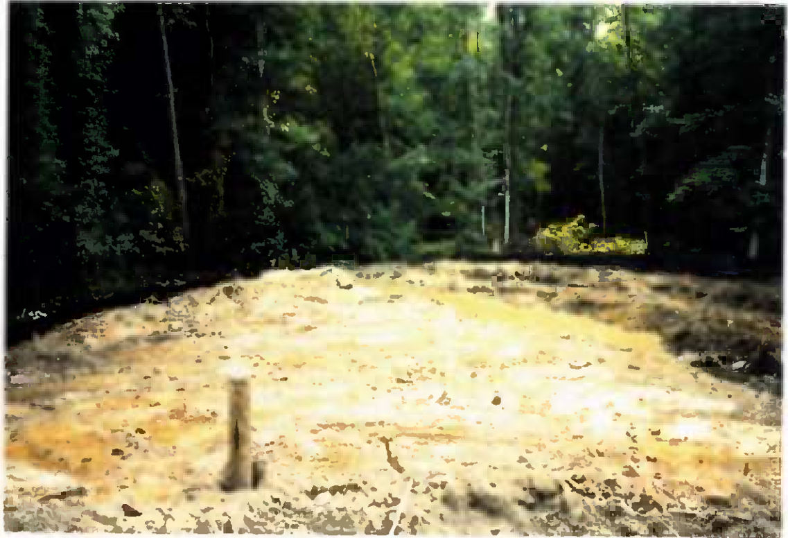
Project No. 16487 Date: 8/14/95 Contract No. N62470-93-D-3032 Delivery Order: 44 Location: Area A and B Description: Erosion control
