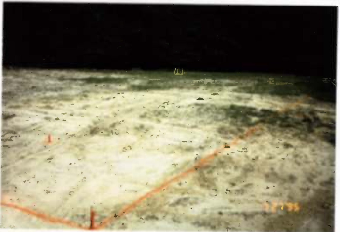
Project No. 16487 Date: 7/27/95 Contract No. N62470-93-D-3032 Delivery Order: 44 Location: Area C Description: Pre-excavation grid
