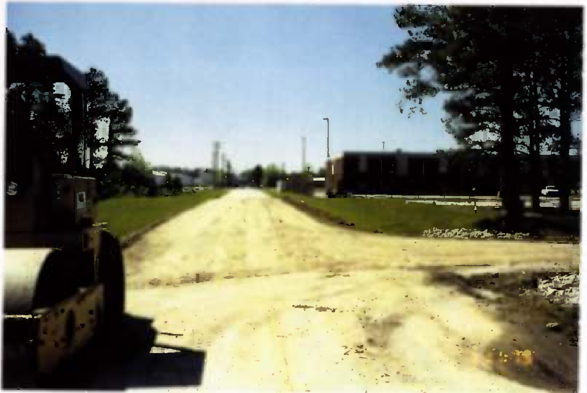
Project No. 16487 Date: 5/1/96 Contract No. N62470-93-D-3032 Delivery Order: 44 Location: Area A and B (roadway) Description: Completed roadway base 'F' Street
