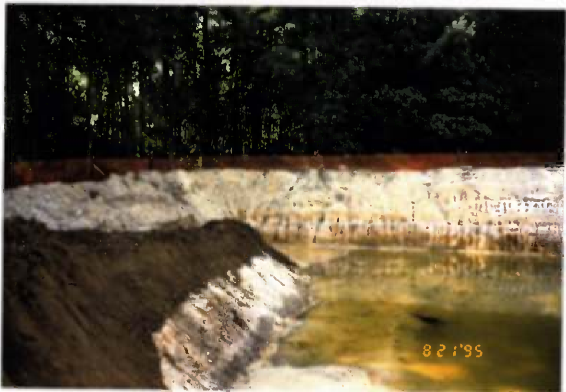
Project No. 16487 Date: 8/21/95 Contract No. N62470-93-D-3032 Delivery Order: 44 Location: Area C Description: Backfilling of Area C
