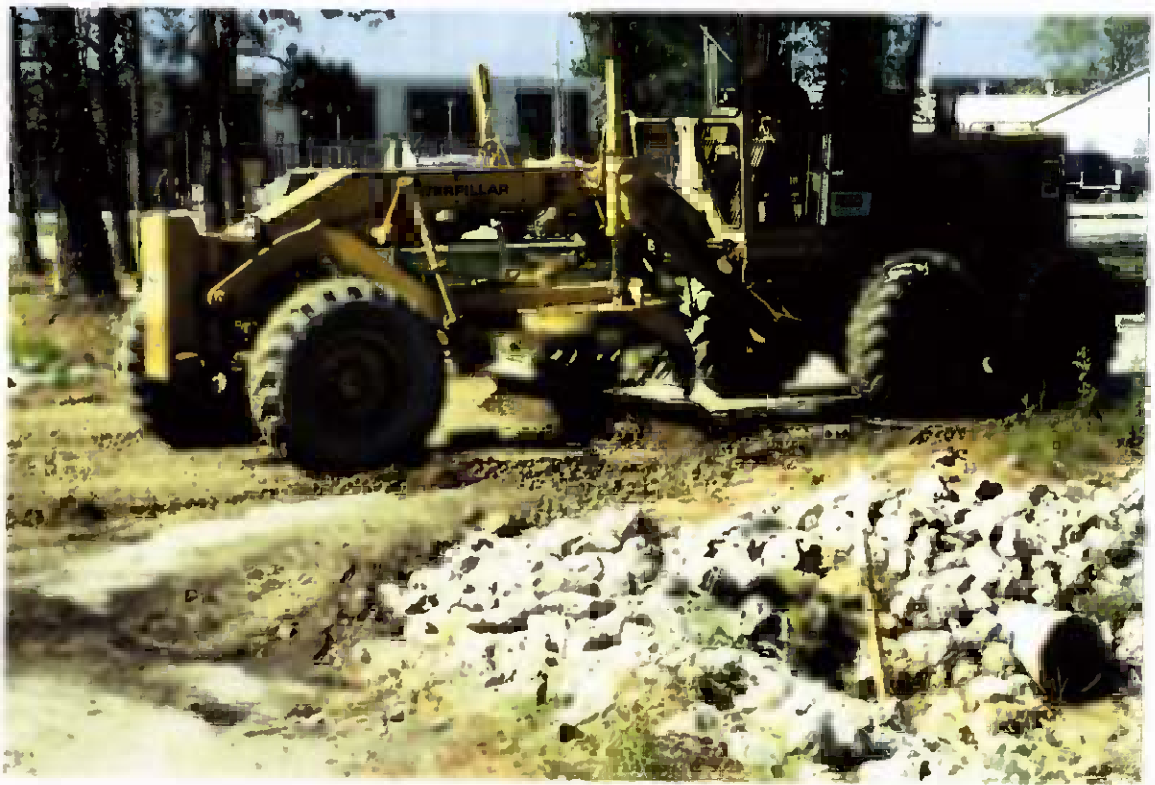
Project No. 16487 Date: 5/1/96 Contract No. N62470-93-D-3032 Delivery Order: 44 Location: Area A and B (roadway) Description: Fine grading
