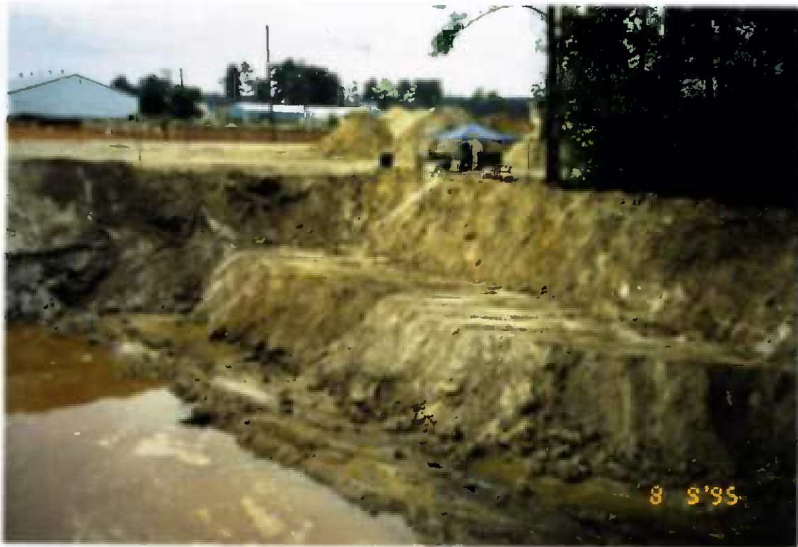
Project No. 16487 Date: 8/9/95 Contract No. N62470-93-D-3032 Delivery Order: 44 Location: Area C Description: Excavation
