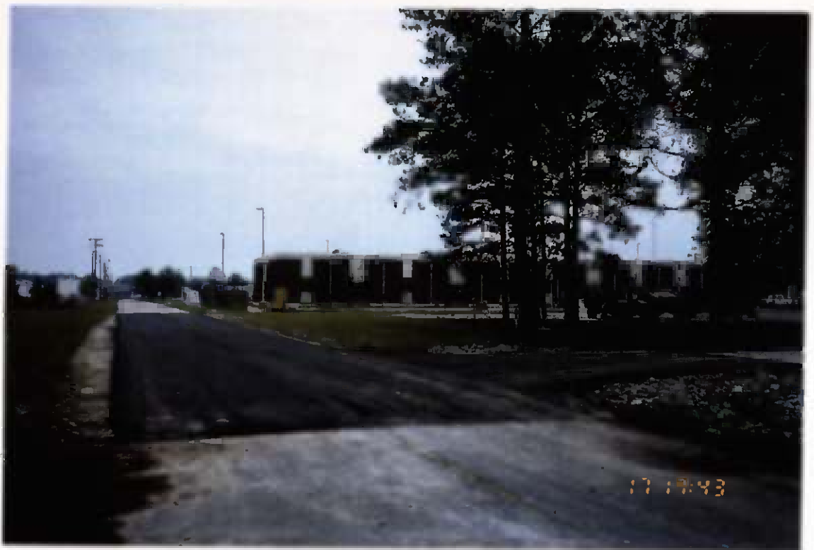
Project No. 16487 Date: 5/17/96 Contract No. N62470-93-D-3032 Delivery Order: 44 Location: Third Street/'F' Street intersection Description: Completed paving
