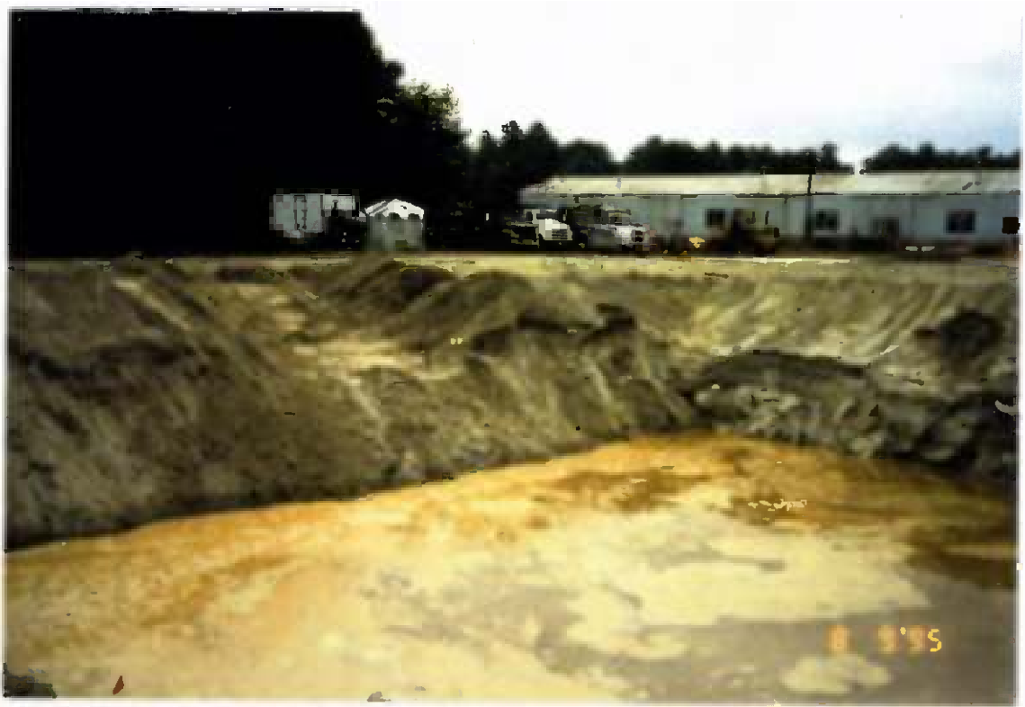
Project No. 16487 Date: 8/9/95 Contract No. N62470-93-D-3032 Delivery Order: 44 Location: Area C Description: Overview of TPH field testing area
