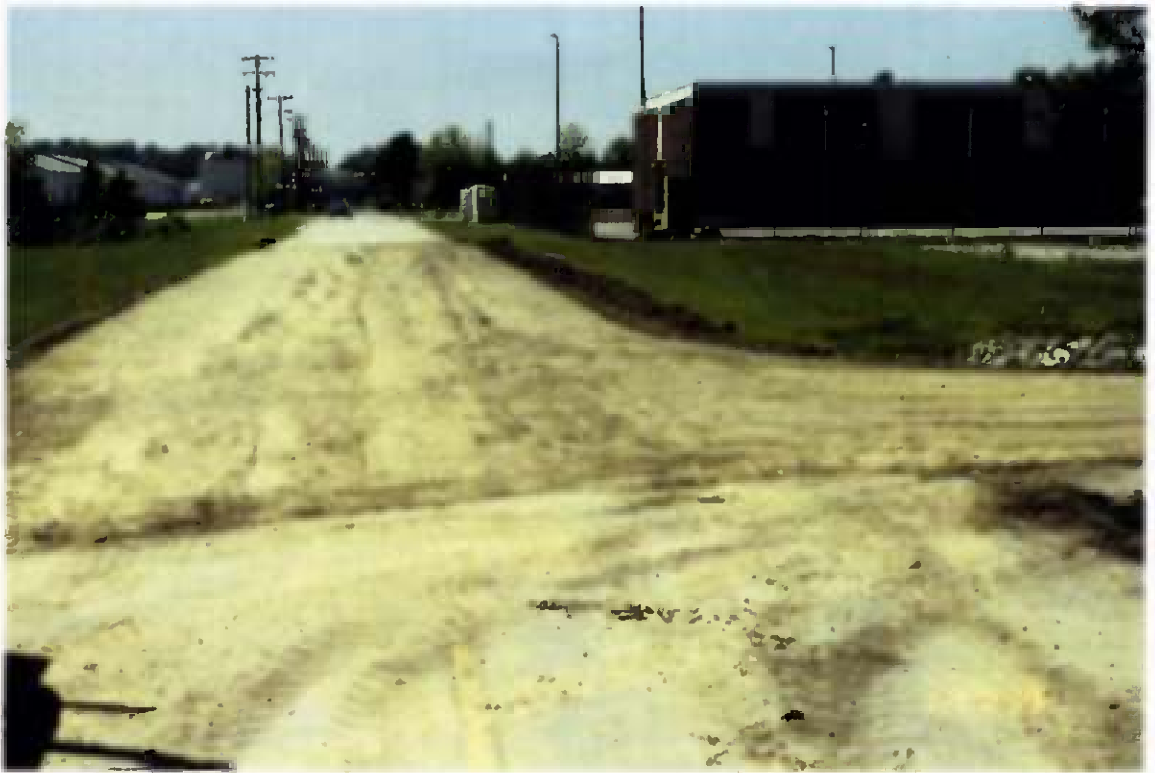
Project No. 16487 Date: 5/1/96 Contract No. N62470-93-D-3032 Delivery Order: 44 Location: Area A and B Description: Completed roadway base 'F' Street
