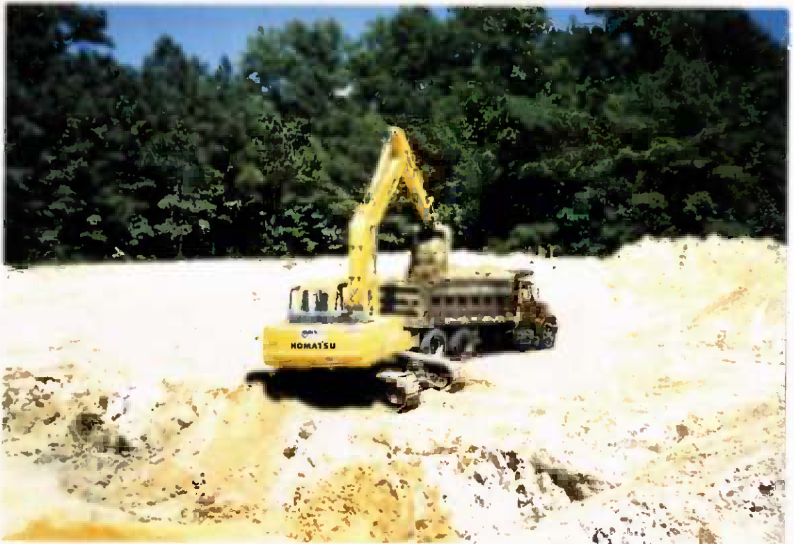
Project No. 16487 Date: 8/4/95 Contract No. N62470-93-D-3032 Delivery Order: 44 Location: Area C Description: Loadout of possible contaminated soil
