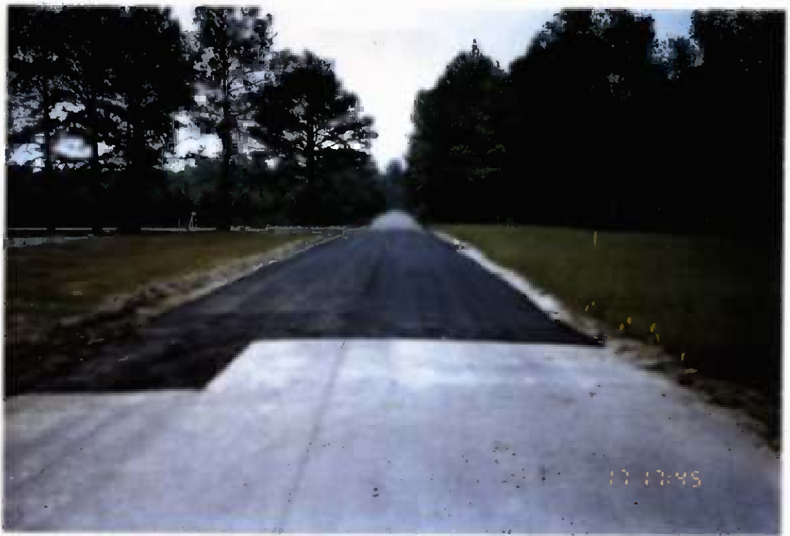
Project No. 16487 Date: 5/17/96 Contract No. N62470-93-D-3032 Delivery Order: 44 Location: 'F' Street - Camp Geiger Description: Completed paving
