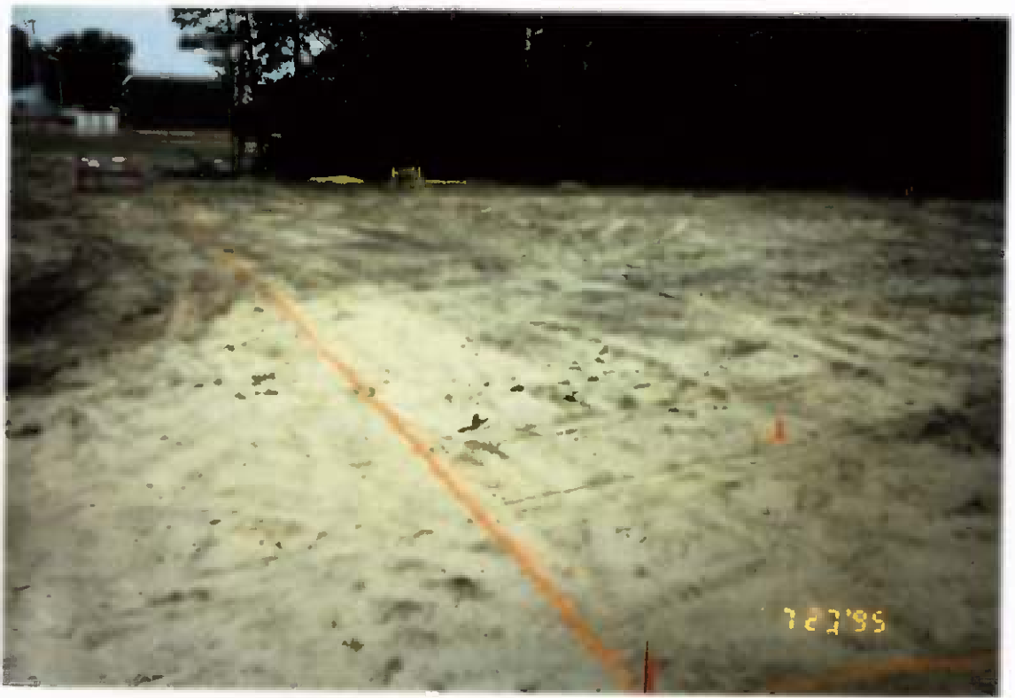
Project No. 16487 Date: 7/31/95 Contract No. N62470-93-D-3032 Delivery Order: 44 Location: Area C Description: Excavation
