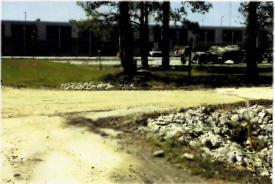
Project No. 16487 Date: 5/1/96 Contract No. N62470-93-D-3032 Delivery Order: 44 Location: Area A and B Description: Completed roadway base 3rd Street
