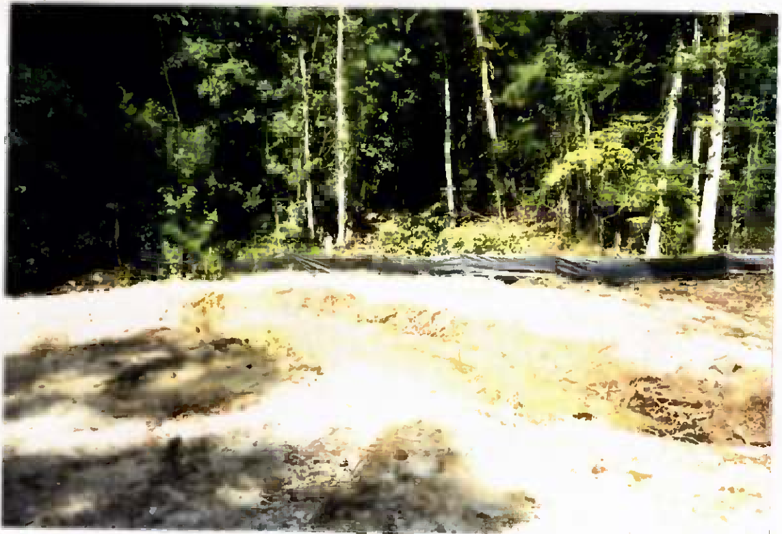
Project No. 16487 Date: 8/9/95 Contract No. N62470-93-D-3032 Delivery Order: 44 Location: Area B Description: Erosion control
