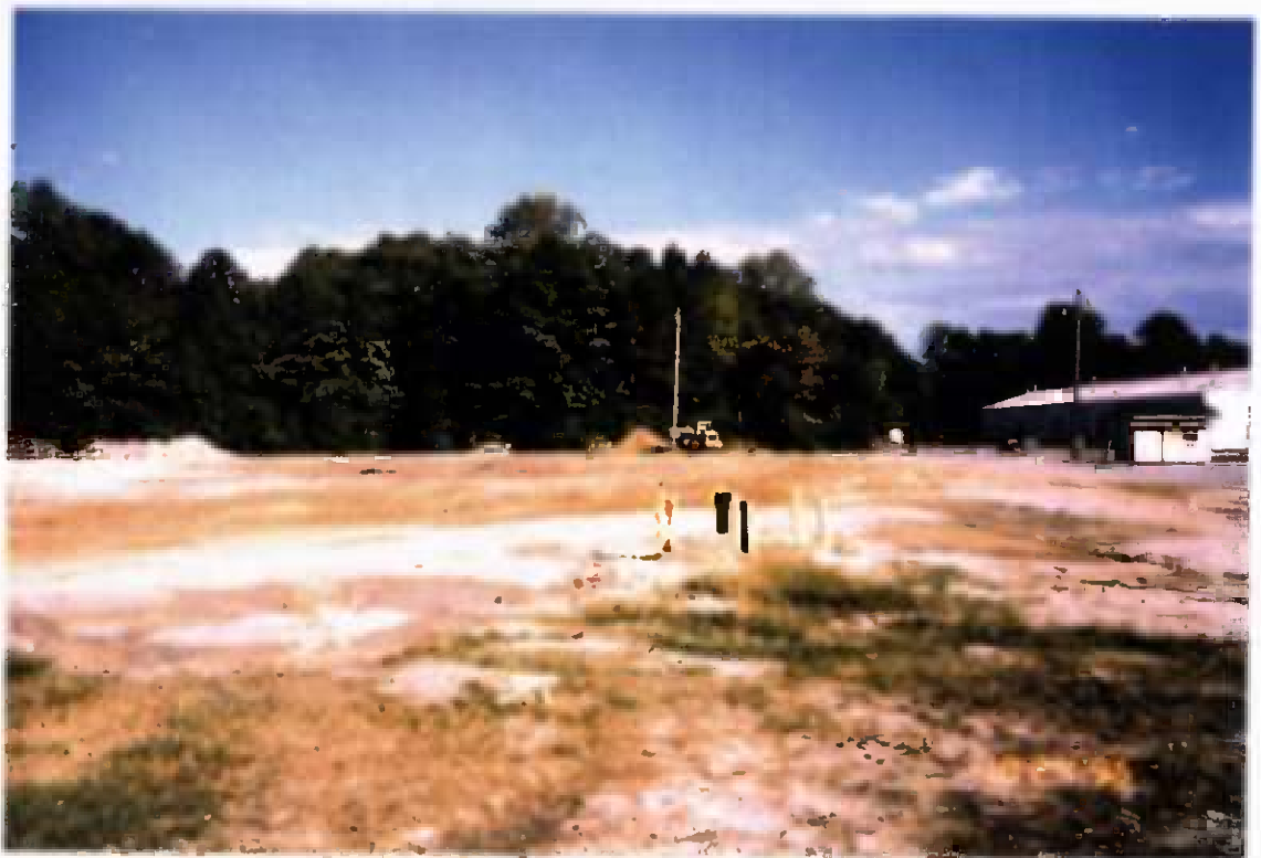
Project No. 16487 Date: 10/24/95 Contract No. N62470-93-D-3032 Delivery Order: 44 Location: Area C Description: Site restoration activities
