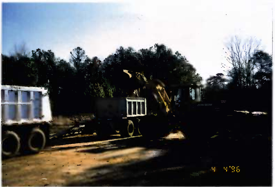
Project No. 16487 Date: 4/4/96 Contract No. N62470-93-D-3032 Delivery Order: 44 Location: Contaminated soil staging area Description: Loading out TPH contaminated soil
