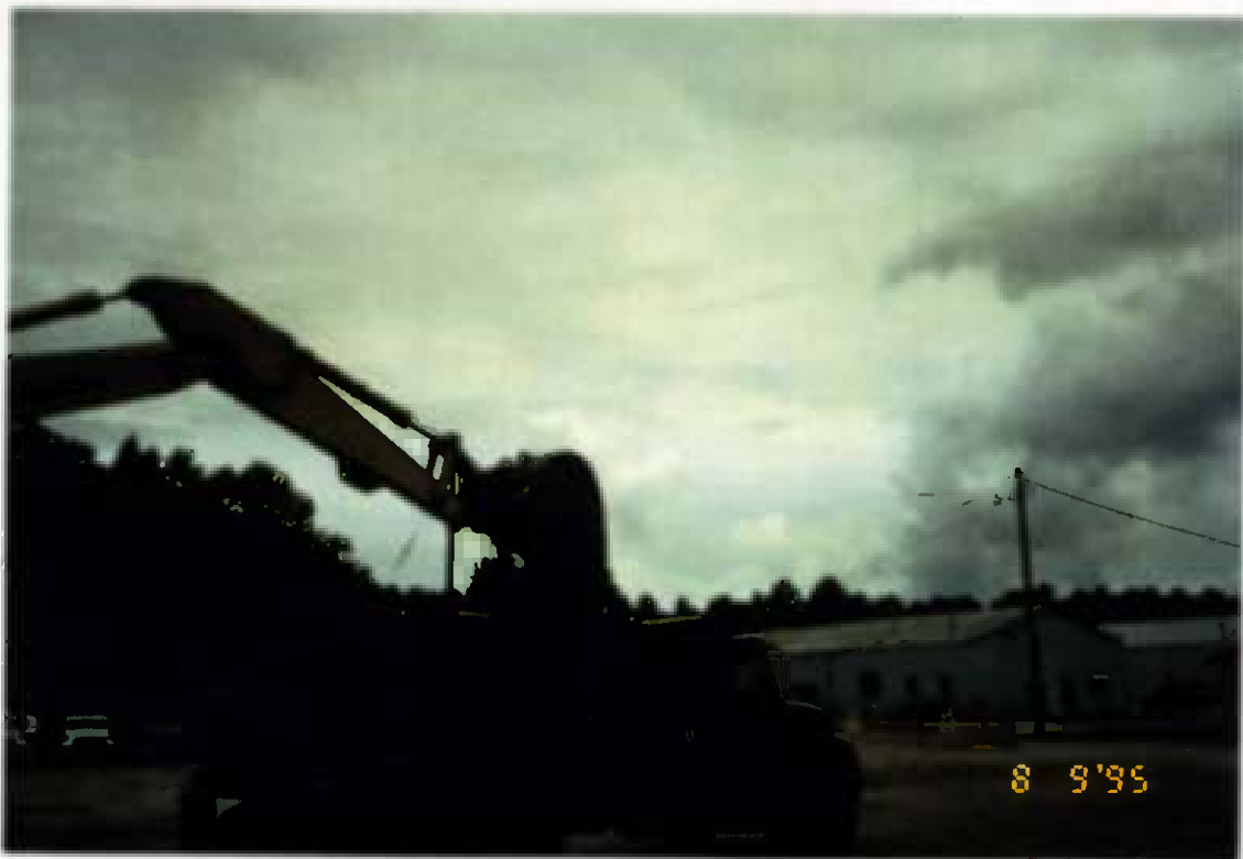
Project No. 16487 Date: 8/9/95 Contract No. N62470-93-D-3032 Delivery Order: 44 Location: Area C Description: Truck loadout
