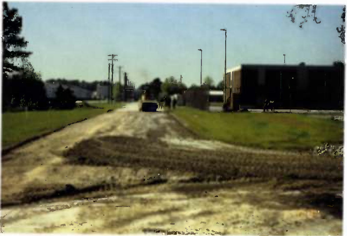
Project No. 16487 Date: 5/1/96 Contract No. N62470-93-D-3032 Delivery Order: 44 Location: Area A and B (road) Description: Road bed preparation
