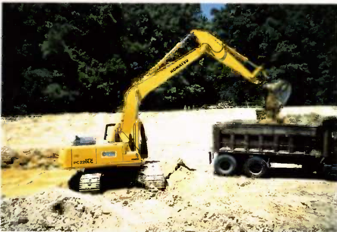
Project No. 16487 Date: 8/4/95 Contract No. N62470-93-D-3032 Delivery Order: 44 Location: Area C Description: Excavation of possible TPH contaminated soils
