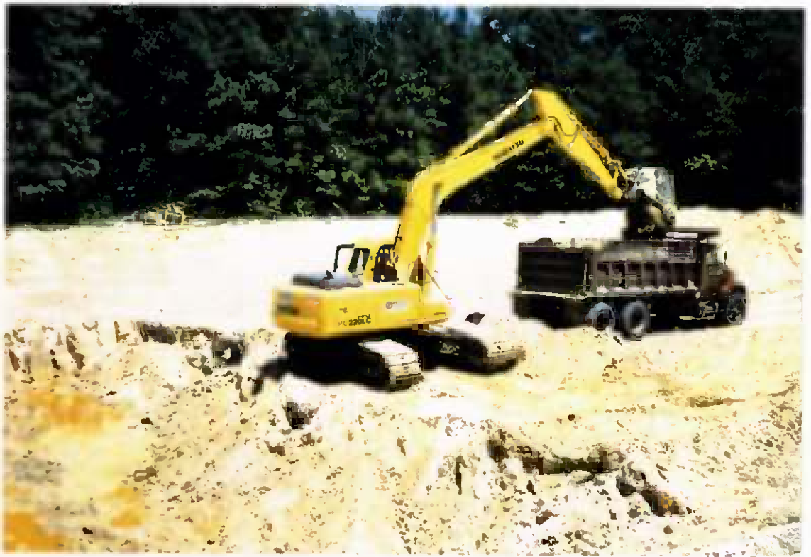
Project No. 16487 Date: 8/4/95 Contract No. N62470-93-D-3032 Delivery Order: 44 Location: Area C Description: Loadout of possible TPH contaminated soil
