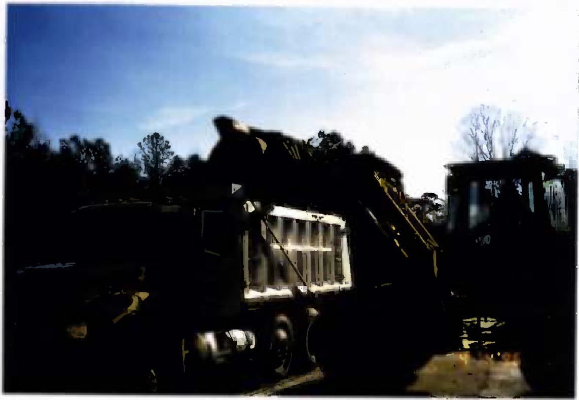
Project No. 16487 Date: 4/4/96 Contract No. N62470-93-D-3032 Delivery Order: 44 Location: Contaminated soil staging area Description: Loading trucks
