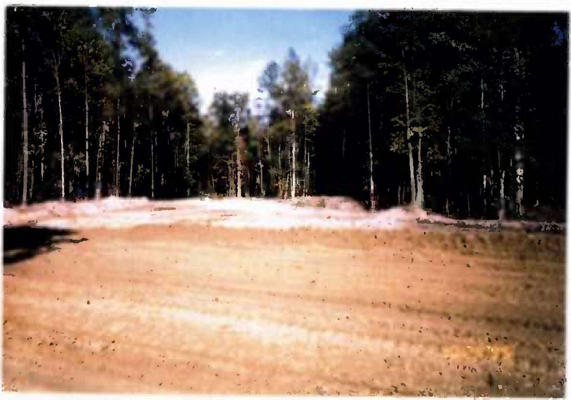
Project No. 16487 Date: 10/24/95 Contract No. N62470-93-D-3032 Delivery Order: 44 Location: Area A and B Description: Backfill of F Street
