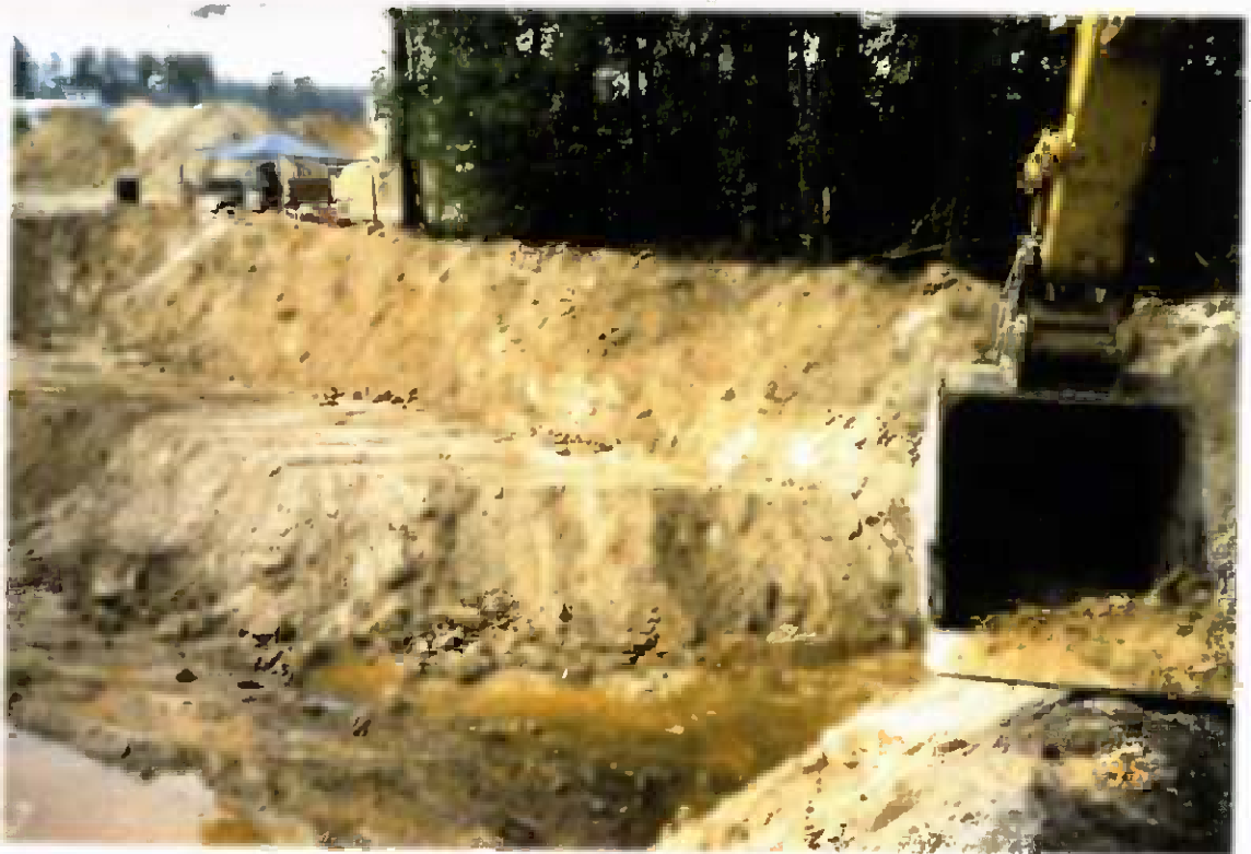
Project No. 16487 Date: 8/9/95 Contract No. N62470-93-D-3032 Delivery Order: 44 Location: Area C Description: Benching excavation
