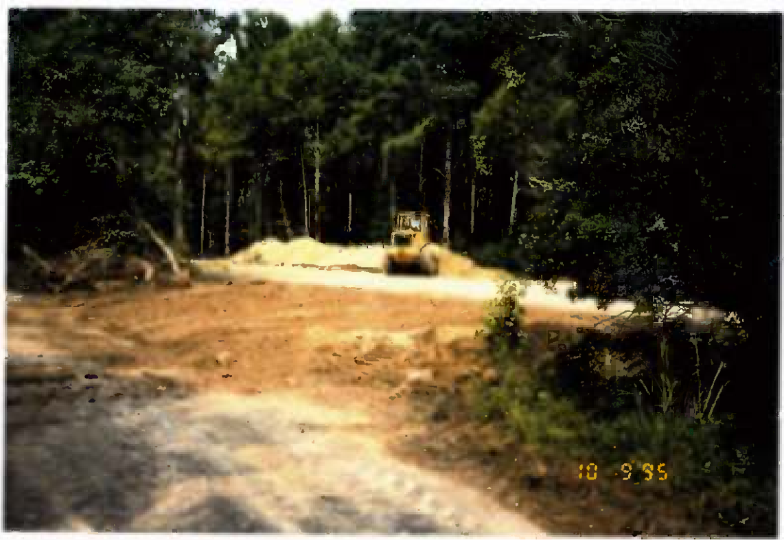
Project No. 16487 Date: 10/9/95 Contract No. N62470-93-D-3032 Delivery Order: 44 Location: Contaminated soil staging area Description: Loading contaminated soils
