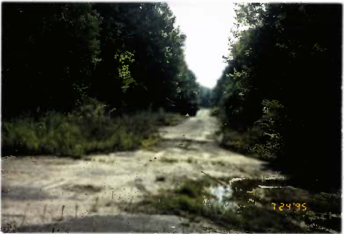
Project No. 16487 Date: 7/24/95 Contract No. N62470-93-D-3032 Delivery Order: 44 Location: Contaminated Stockpile Area Description: Site Prep
