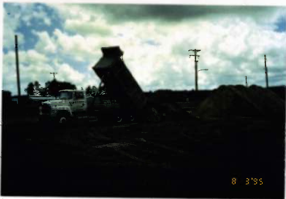
Project No. 16487 Date: 8/3/95 Contract No. N62470-93-D-3032 Delivery Order: 44 Location: Area C Description: Clean soil staging area
