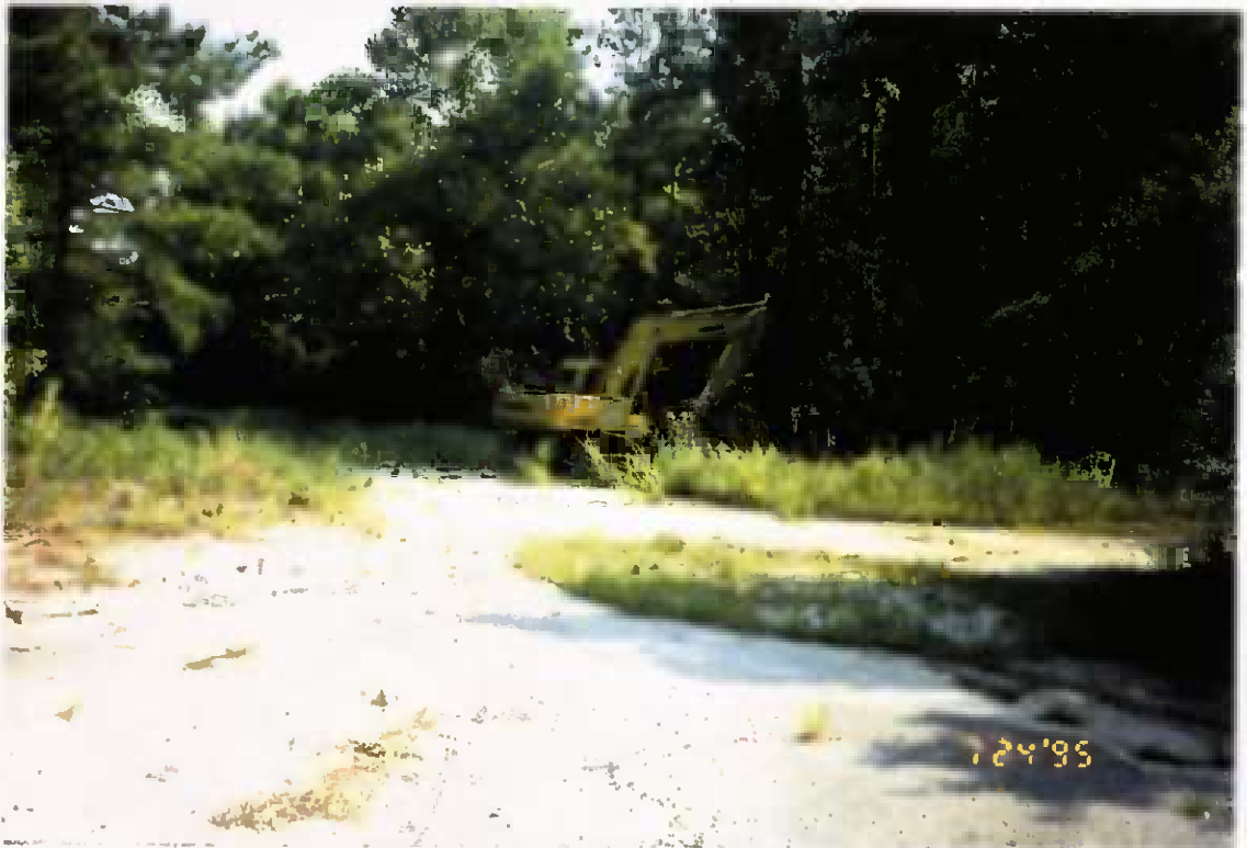
Project No. 16487 Date: 7/24/95 Contract No. N62470-93-D-3032 Delivery Order: 44 Location: Contaminated Stockpile Area Description: Site Prep
