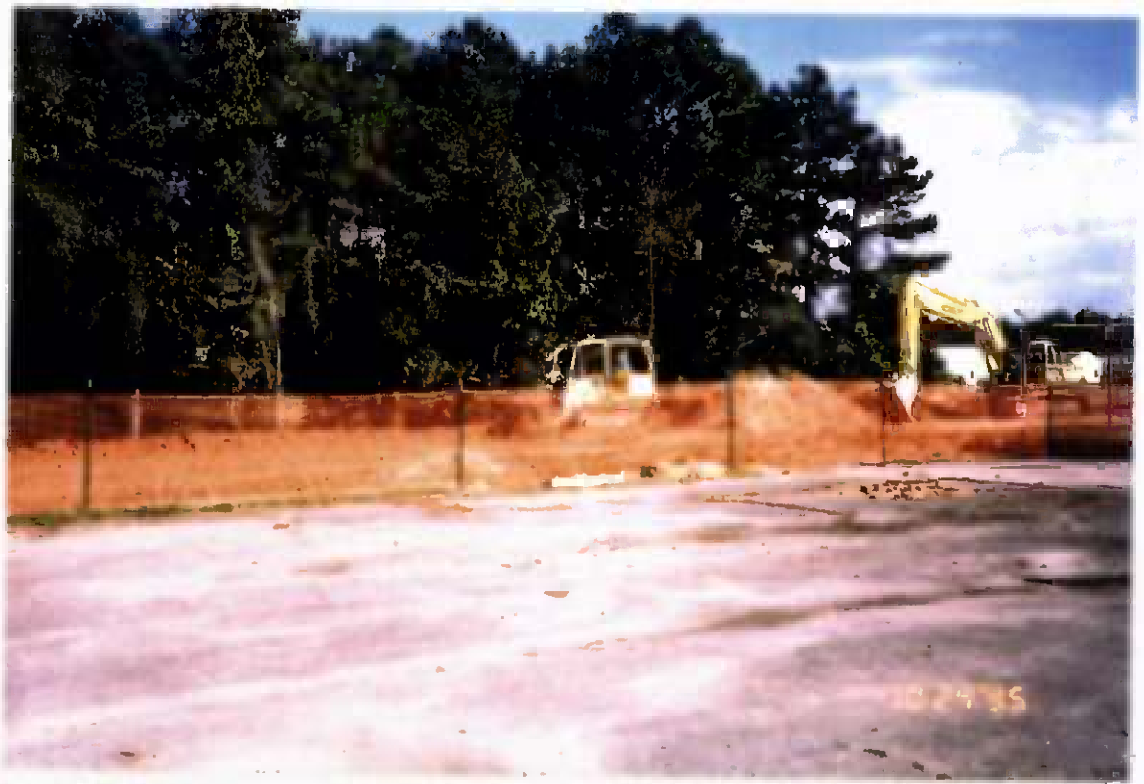
Project No. 16487 Date: 10/24/95 Contract No. N62470-93-D-3032 Delivery Order: 44 Location: Area A Description: Backfill of Area A
