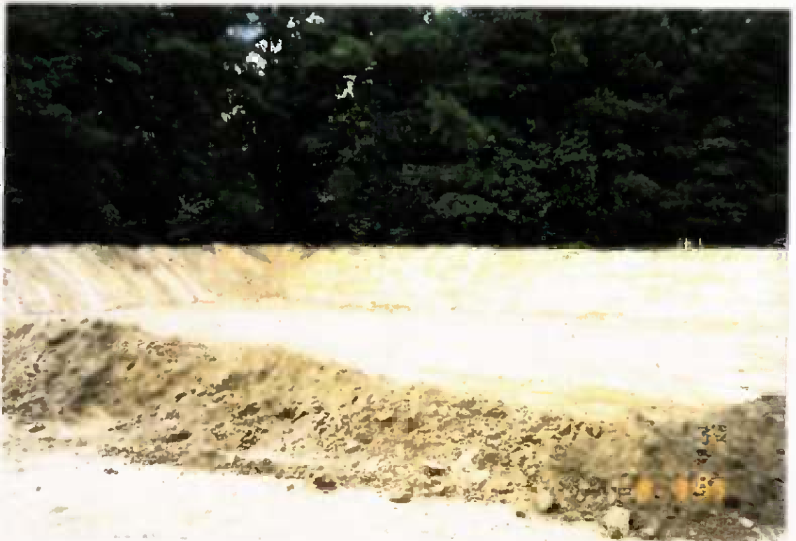
Project No. 16487 Date: 8/3/95 Contract No. N62470-93-D-3032 Delivery Order: 44 Location: Area C Description: Area C excavation
